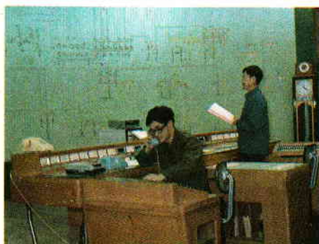
The control room of the Guizhou power grid. Zhou Youma
