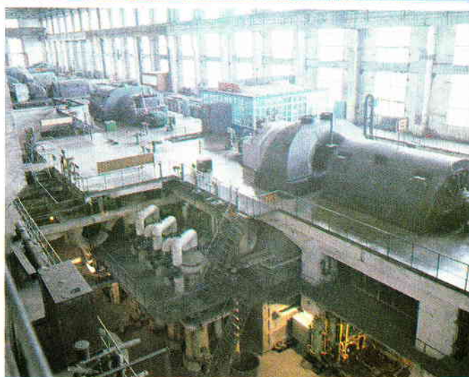
Turbogenerators in the Qingzhen thermal power plant. Zhou Youma
